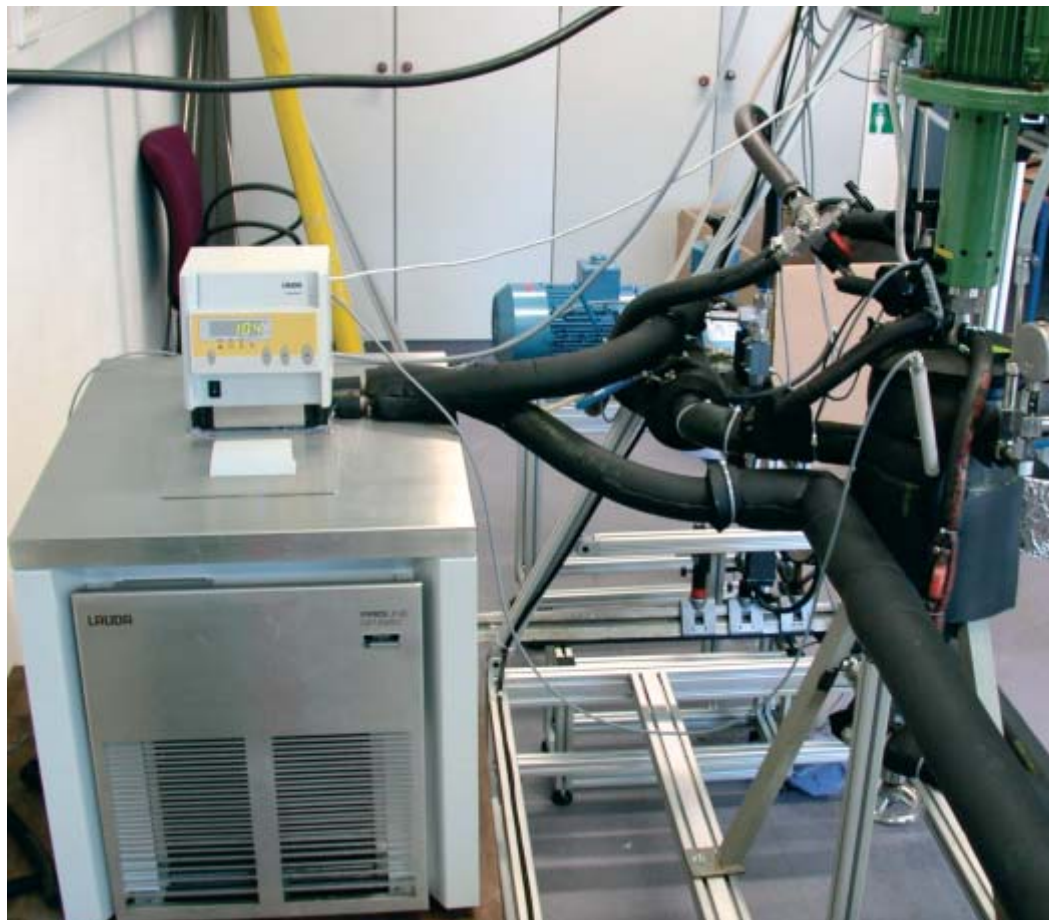
Connections of the LAUDA Proline RP 890 C to the reactor system.
